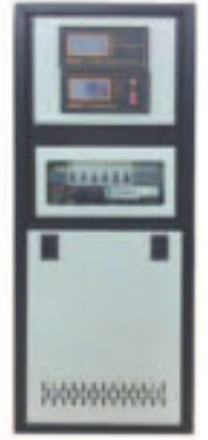
ASC-2426 TOWER 24VDC 26AH REDRESÖRLER
